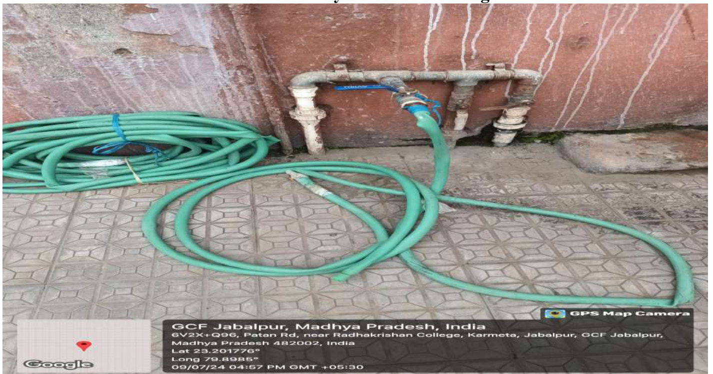
Bore well facility available in college
